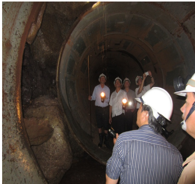
Fig.6. The second damage of penstock
