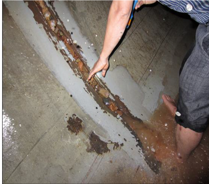
Fig. 5. The first damage of penstock
